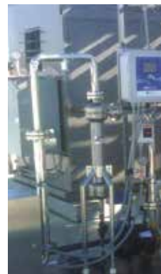
ILS used to remove solids from water supply system for a large grocery store.
