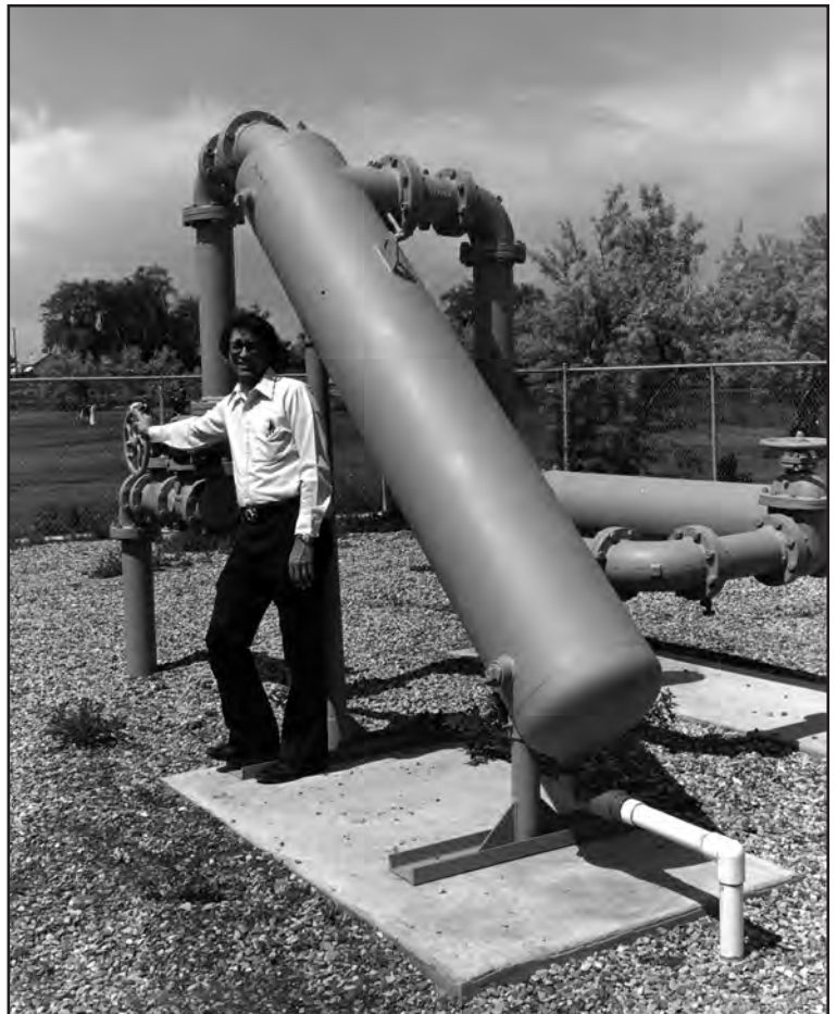
Carl R. Nelson, Jr. stands beside Lakos Separator installation at Mick Riley Golf Course, Salt Lake City. Drawn from lakes, water is pumped through screen and Lakos unit to sprinkler system.
