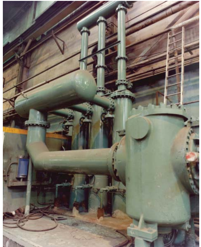
Three vertical profile LAKOS RFD Separators at work in the plate mill.
