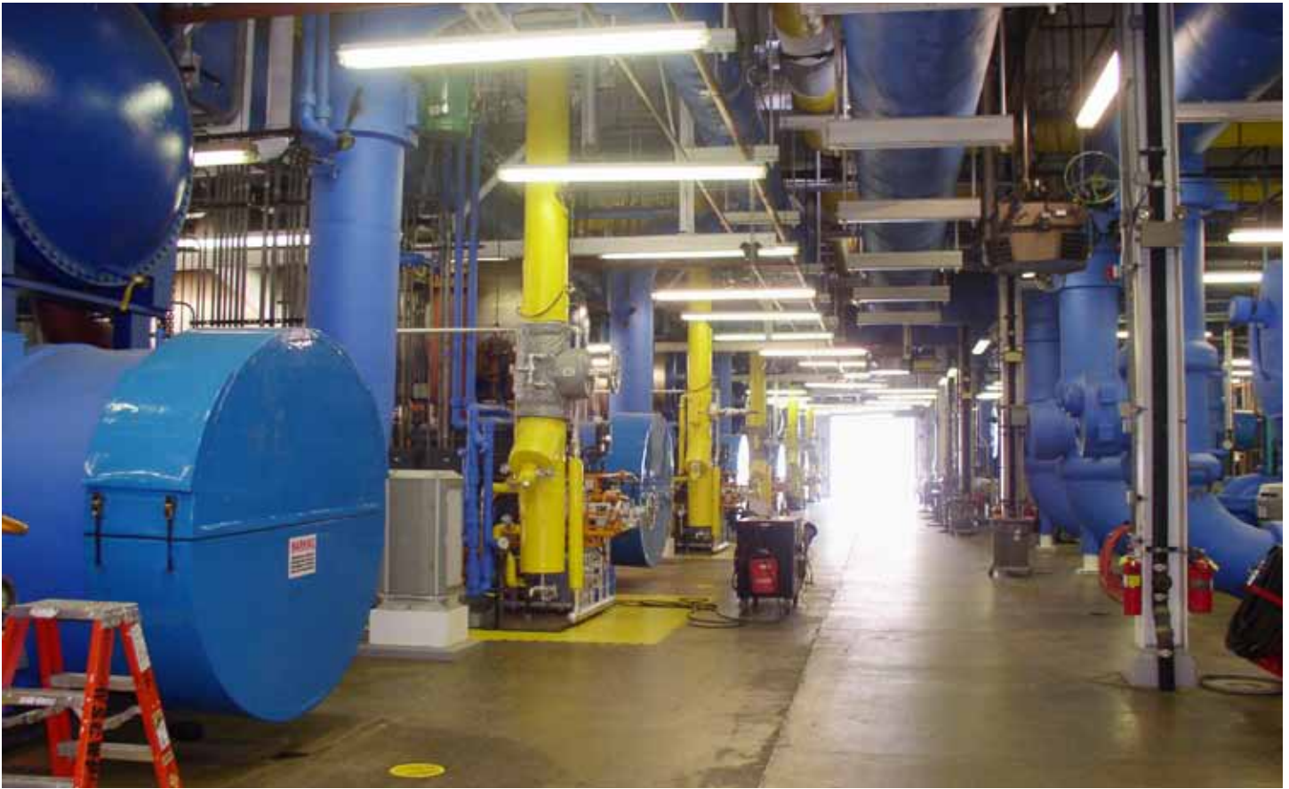
Chillers at Citizens Thermal West Street chilled water plant
