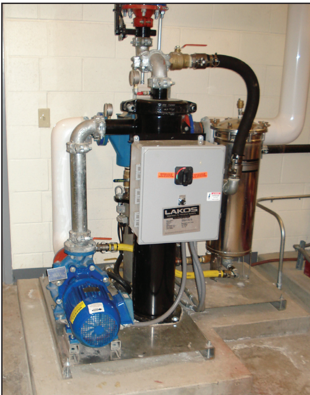
Left: LAKOS SPX-0145-SRV as a side-stream filtration unit on the Joe Crowley Student Union at UNR
