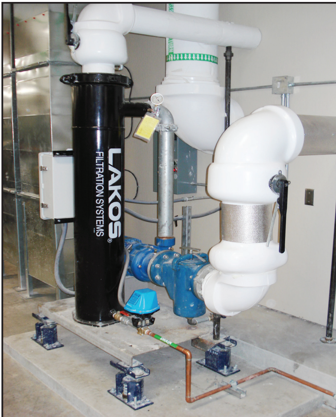
LAKOS TCX-0280-ABV basin sweeping filtration unit installed at the Mathewson - IGT Knowledge Center at UNR
