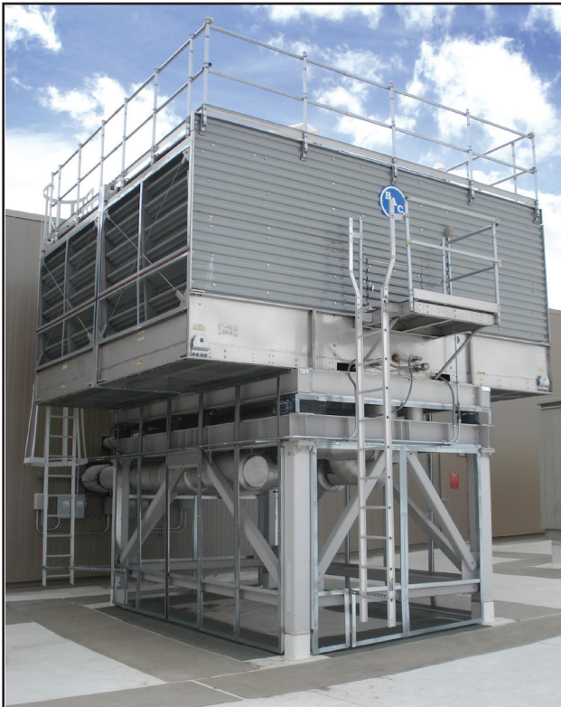
Above: Cooling Tower at UNR Mathewson - IGT Knowledge Center at UNR
