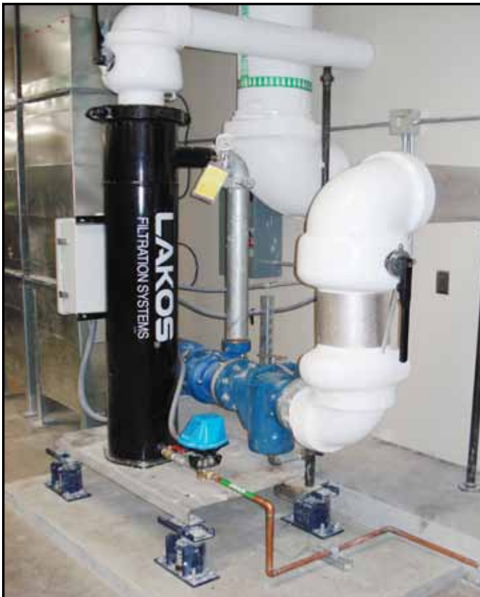
LAKOS TCX-0280-ABV basin sweeping filtration unit installed at the Mathewson - IGT Knowledge Center at UNR
