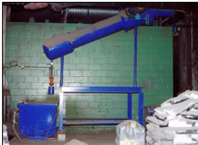
LAKOS PREP System helps solve Lukens Steel's waste problems by separating and transferring highly concentrated scale from hotwell; sludge purged into LAKOS Solids Collection Hopper.
