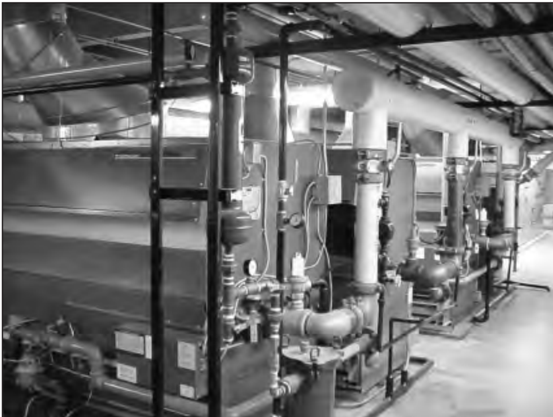
LAKOS - Boiler loop installation - supply connection {side-stream}
