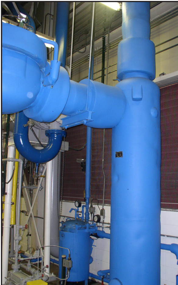
LAKOS RTS 1209 Separator has been working at Citizens Thermal West Street chilled water plant since 1992
