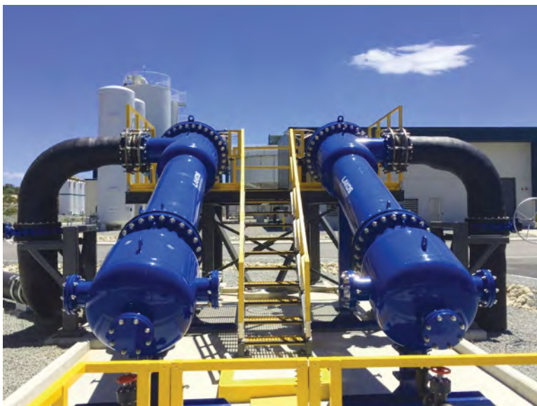
Two JSK Separators installed at a desalination plant
