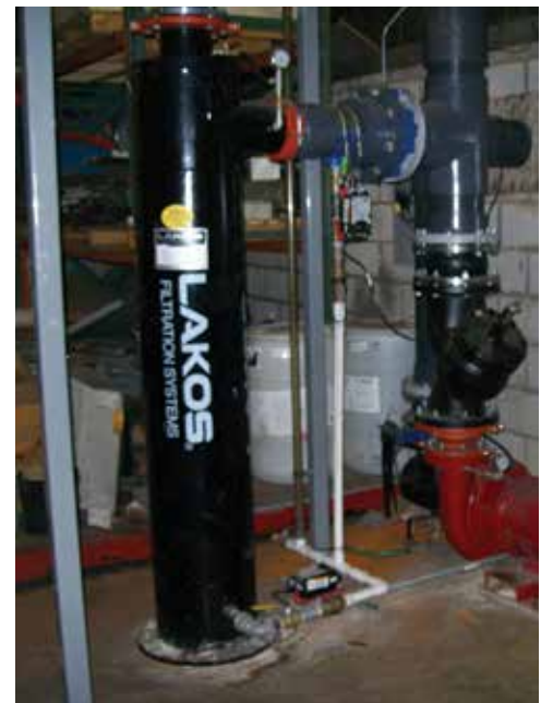
LAKOS HTH 0500 used to keep water tower condenser free of solids in chilled water system.
