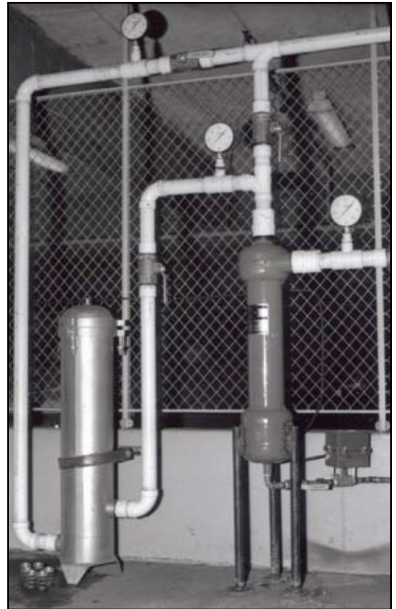
As shown here, a Lakos In-Line Separator pre-filters each of their four cartridge filters. Note the cartridge bypass piping, needed when servicing the cartridges ... and unnecessary with the automatic Lakos units.
