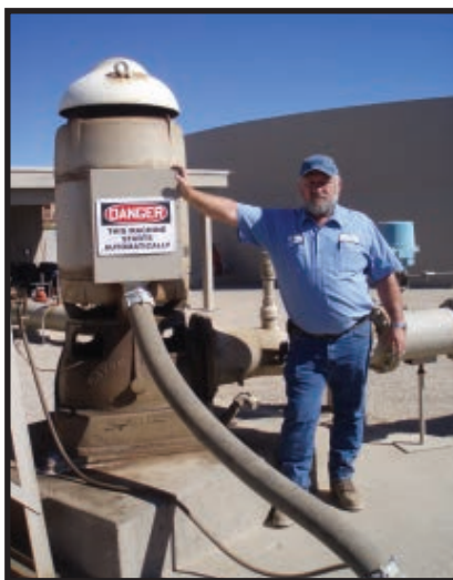
Ron Baysinger of Queen Creek Water Company next to one of nine LAKOS protected turbine pumps.
