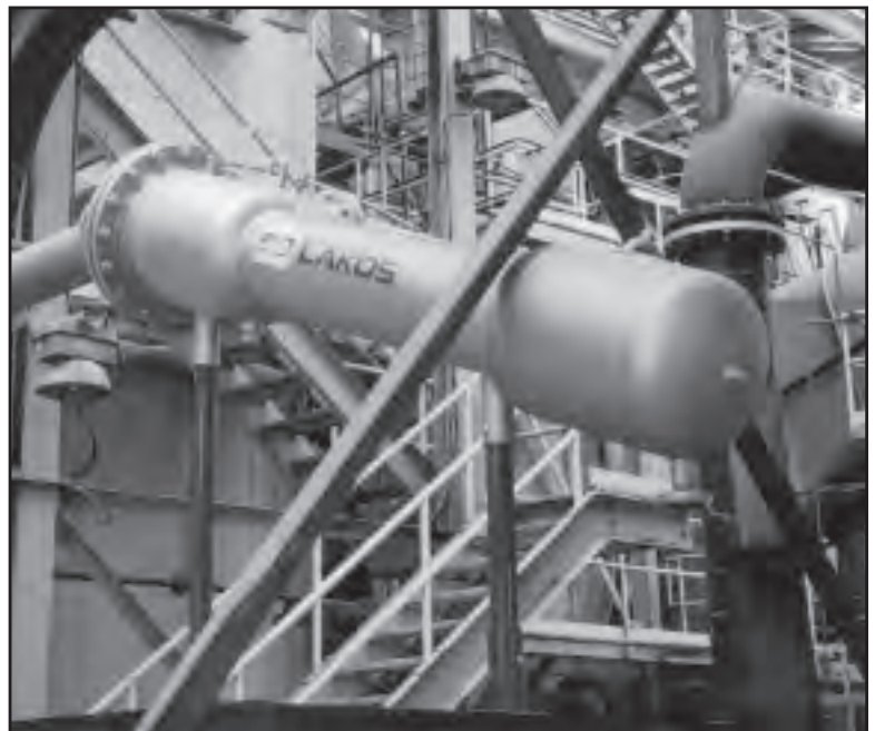
One of four stainless steel LAKOS PRX Separators installed at Magma Copper Company.
