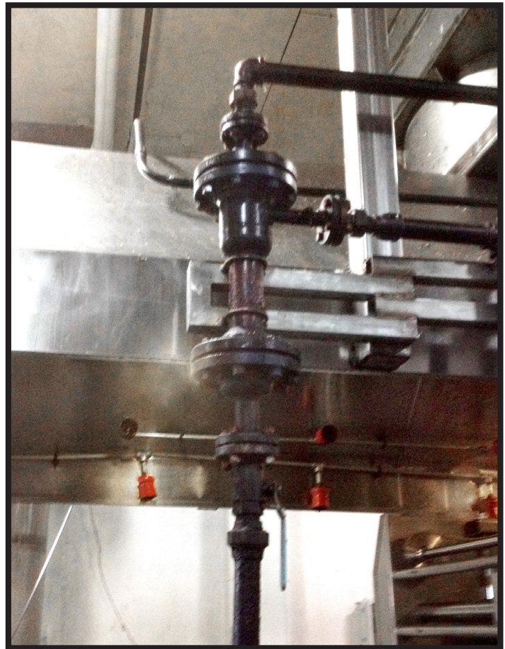
The LAKOS CSX separators cut labor costs in half, saving the snack food company over $60,000 annually.
