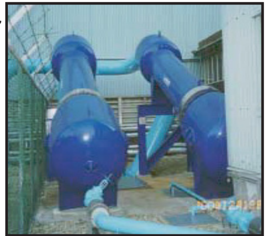
The LFD-2402-B/SK Separators are installed on the seawater intake pumps to protect the heat exchangers from fouling by removing sand, silt, shells and other debris found in sea water. The customer is using 4" pneumatic pinch valves to purge the separators.
