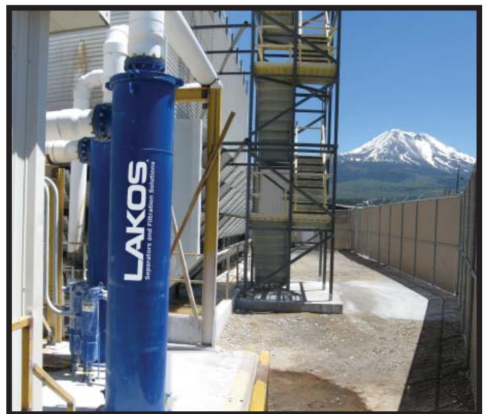
Two LAKOS JPX Separators protect the system despite facing the harsh weather conditions of Northern California.
