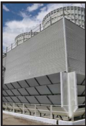
The Cogen system's cooling tower basin is exposed, making it vulnerable to dirt and debris.
