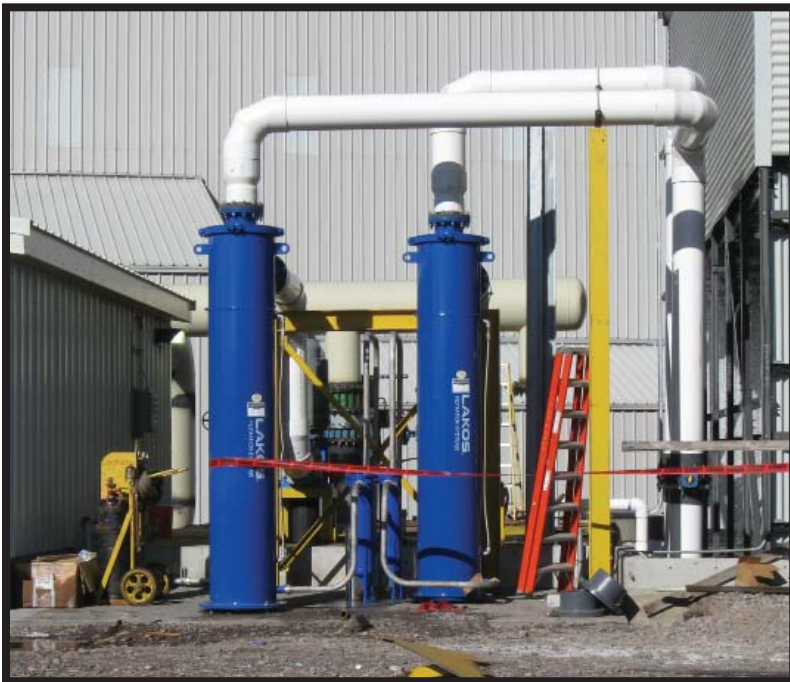
LAKOS JPX Separators during installation.
