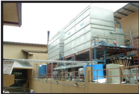
The hotel's cooling towers are only 50 feet away from the beach, making solids-free water a top concern
