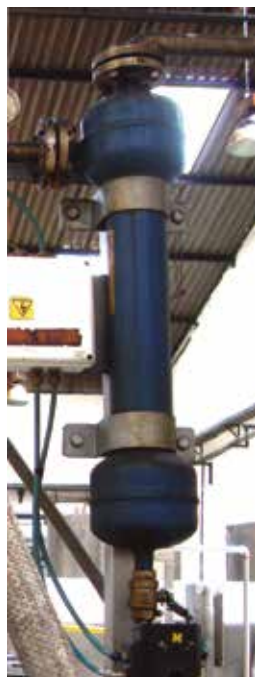
ILB removes solids in a food processing plant.
